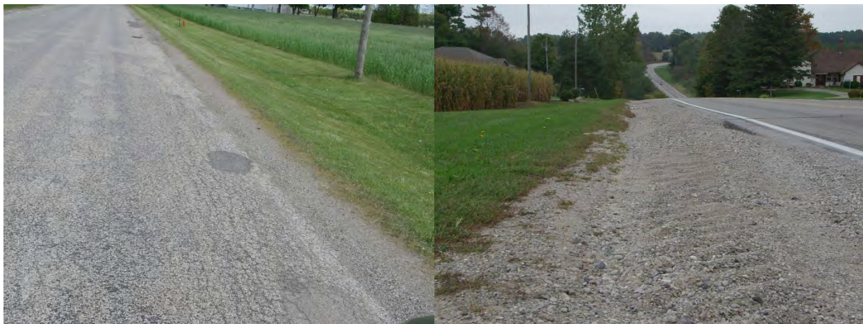
Figure 14 Shoulder Berm Contributing to Edge Failure
