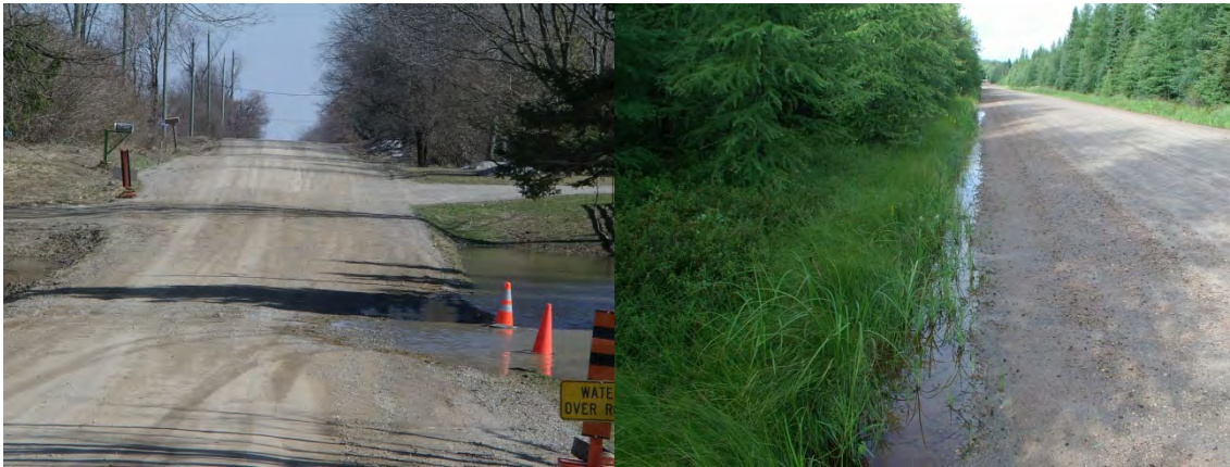
Figure 13 Inadequate Roadside Drainage
