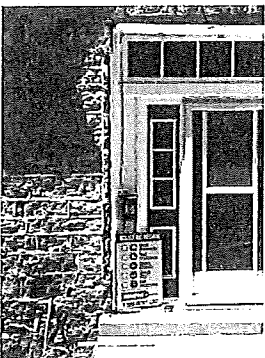
This photo shows the attempt to make the storm porch as air-tight as possible during the winter months when the windows were in place.
