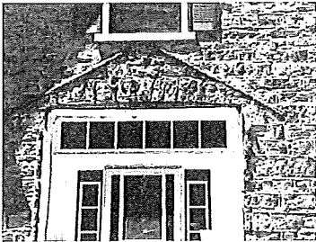
This photo shows the foam on the stonework that had been injected along the old porch windows
