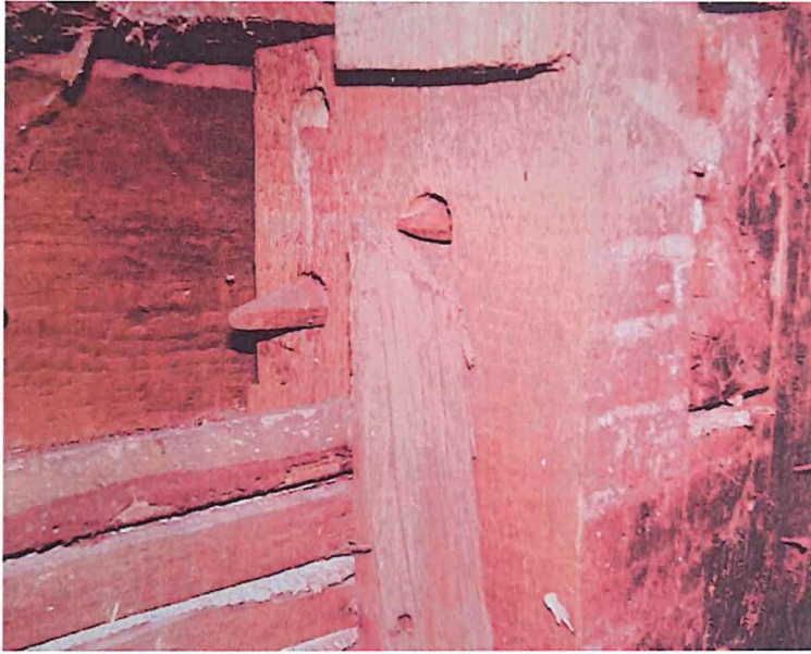
Figure 8: Tree nail construction located in the rear north side of the house shown in a 2005 photograph.
