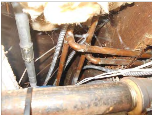
Presumed lead-containing solder present on pipes in the building.
