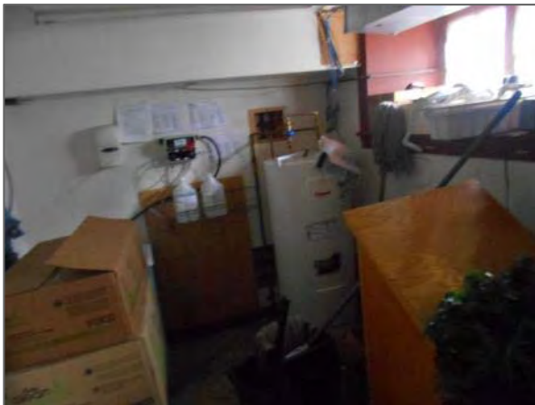
Hot water tank insulated with non-asbestos fiberglass.
