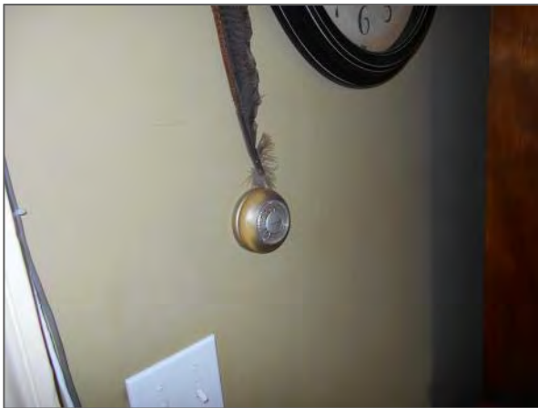
Mercury containing thermostat present in the building.
