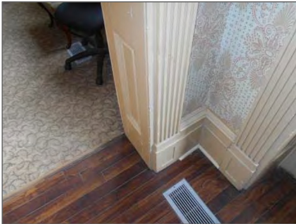
Yellow painted wood trim containing elevated concentrations of lead (>1,000 ug/g).
