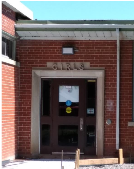
175 William Street South, former girls entrance viewed from the west (E. Tumak, August 2019).
