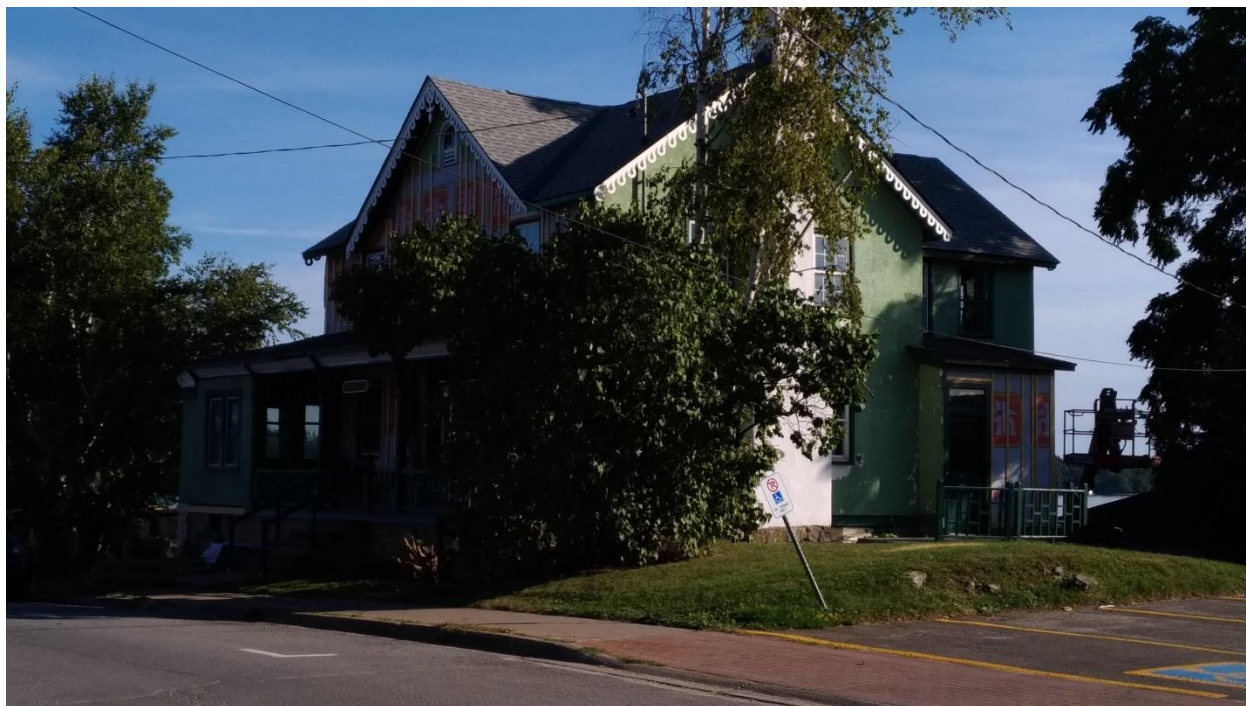
588 Stone Street South, viewed from the northeast during renovations after removal of vinyl siding (E. Tumak, Sept. 2019).
