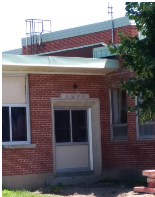
175 William Street South, former boys entrance viewed from the west (E. Tumak, August 2019).
