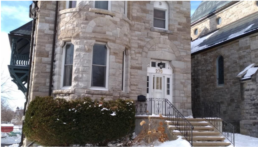
Figure 27: Detail of ground level windows and main entrance of the rectory (E. Tumak, Jan. 2020).
