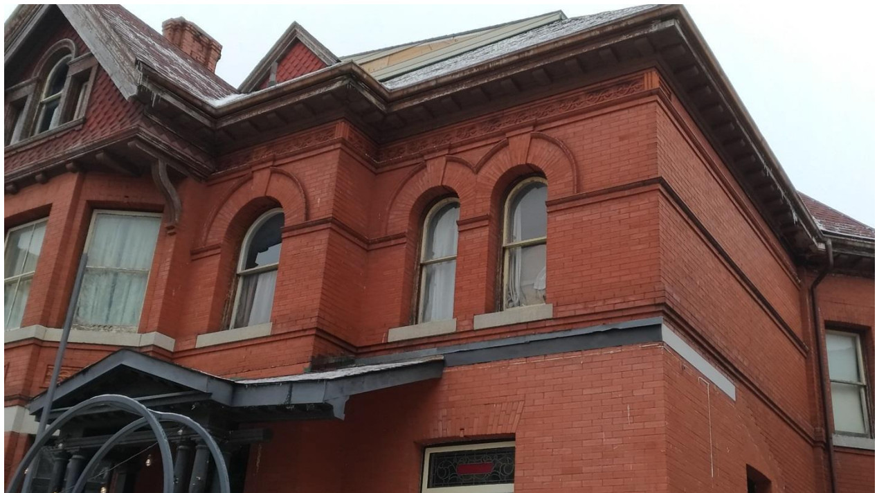
Figure 18: Detail of the second level windows at the west side of the front, highlighting the voussoirs and the terra cotta panels above (E. Tumak, Jan. 2020).
