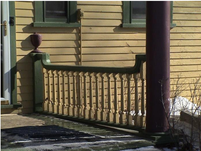
Figure 13. 95 King St. W., Gananoque, porch detail at the southeast/rear end of the building. Photo: Edgar Tumak, Jan., 2008.
