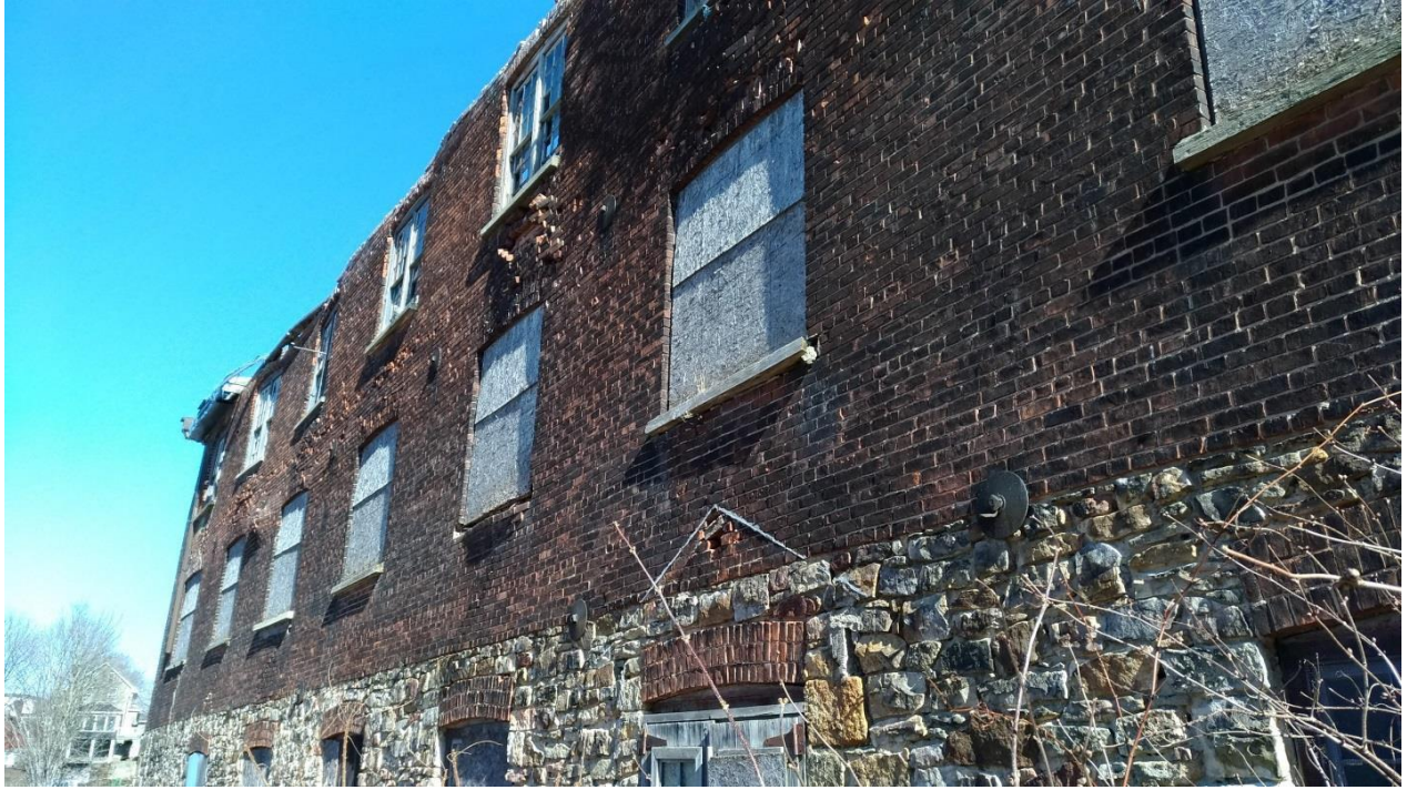
Figure 14: Brick Building, viewed from the northwest, showing the deterioration and bowing of the northeast wall (E. Tumak, March 2020).
