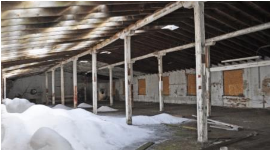
Figure 15: Brick Building upper level interior looking east, showing the breach in the roof at the northeast end as early as 2014, and the resulting moisture/snow infiltration (source, "185 Mill Street and 15 Clarence Street" Heritage Impact Statement, March 2014, Appendix A, p. 28).
