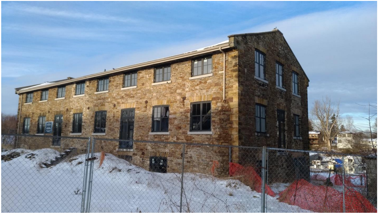
Figure 4: 185 Mill Street, Stone Building, viewed from the southwest after recent renovation interventions affecting the fenestration and entrances (E. Tumak, Jan. 2020).
