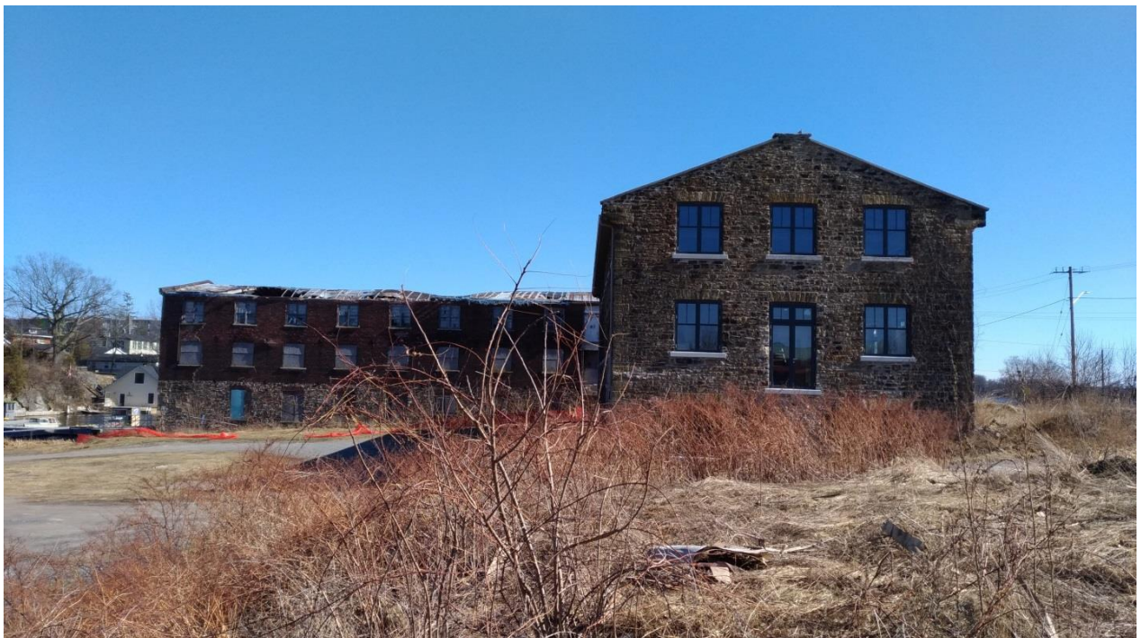
Figure 13: View from the north, showing the partially collapsed north roof of the Brick Building (E. Tumak, March 2020).
