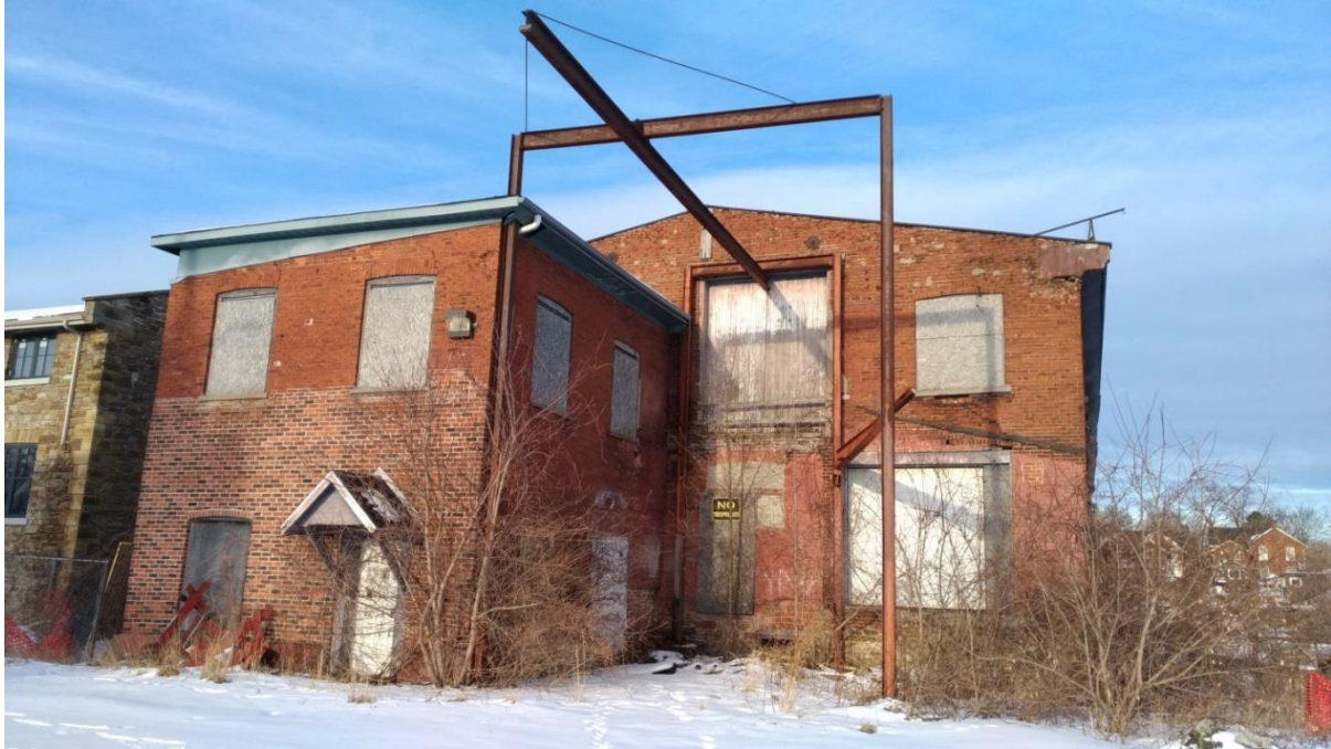
Figure 8: 185 Mill Street, Brick Building, west elevation. The two-storey brick extension in the foreground dates from ca. 1895-1900. (E. Tumak, Jan. 2020).
