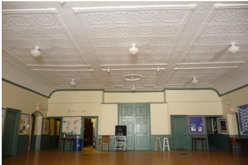
Figure 6: St. Andrew’s, Gracey Hall looking west toward the church, showing the decorative, pressed metal ceiling (photo E. Tumak, May, 2015).
