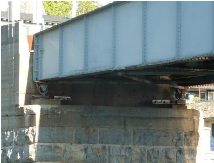
Figures 4-5: left – detail of the east abutment of the Gananoque Swing Bridge, viewed from the northwest; below middle – east abutment and stepped protective embankment of the Gananoque Swing Bridge, viewed from the northwest; and below bottom – view from the bridge looking north up the Gananoque River showing the bridge deck steel grill of the vehicle lane and one of the stiffening side plates (photo E. Tumak, Sept. 2013)
