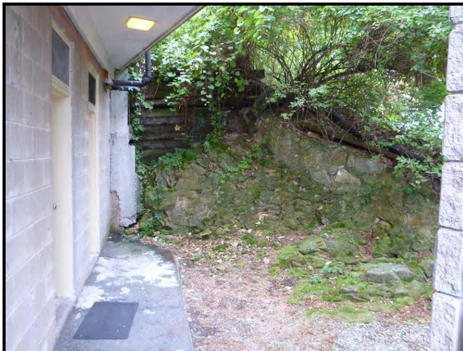
Figure 28. Wood cribbing and stone wall along the eastern property boundary, looking north. (PR13-D07)
