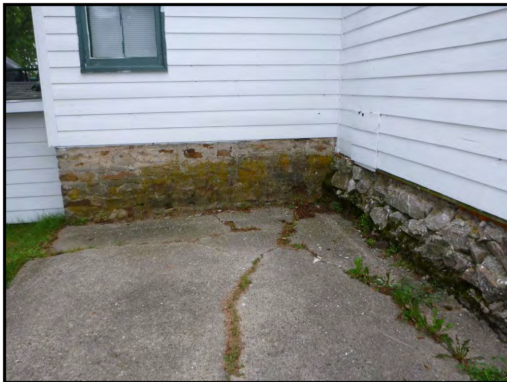
Figure 22. View of the east side of the dwelling at 119 South Street showing the stone foundation, looking southwest. (PR13-24D18)
