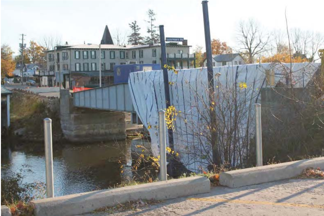
Image 12: The Water Street Swing Bridge has been listed by the Town of Gananoque pursuant to Section 27 of the Ontario Heritage Act .
