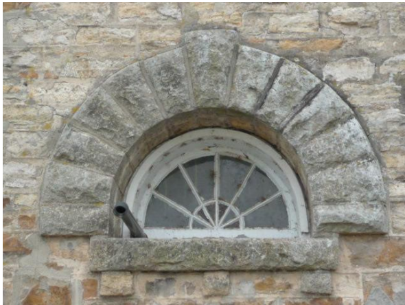
Figure 5: left – Gananoque Pump House, window detail of the northeast/Kate Street elevation (photo E. Tumak, July 2009).
