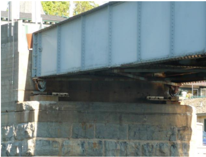
Figures 4-5: left – detail of the east abutment of the Gananoque Swing Bridge, viewed from the northwest; below middle – east abutment and stepped protective embankment of the Gananoque Swing Bridge, viewed from the northwest; and below bottom – view from the bridge looking north up the Gananoque River showing the bridge deck steel grill of the vehicle lane and one of the stiffening side plates (photo E. Tumak, Sept. 2013)
