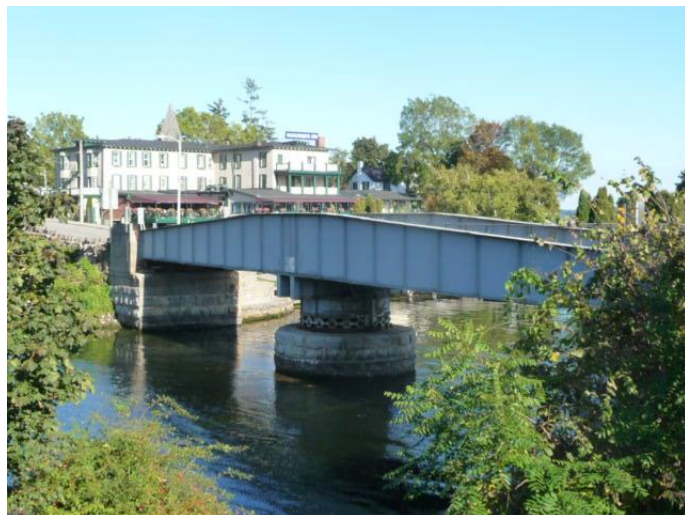
Figure 1: Gananoque Swing Bridge, viewed from the northwest, with the Gananoque Inn in the background (photo E. Tumak, Sept. 2013).
