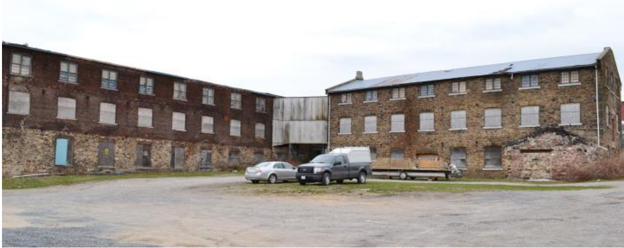
Fig. 4: View of rear. Note location of earlier addition. [actual source: 185 Mill Street, viewed from the northeast, prior to renovation interventions, with the Stone Building on the right/north and the Brick Building on the left/south (Mark Thompson Brandt Architect and Associates, Peer Review: Heritage Impact Statement, ``Mill St. & Clarence St. Development, 'Riverstone,' Gananoque, ON,`` 2014)].
